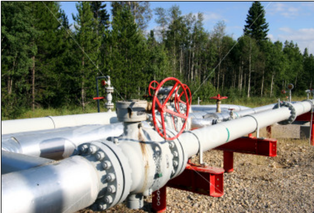
Natural Gas Pipeline
