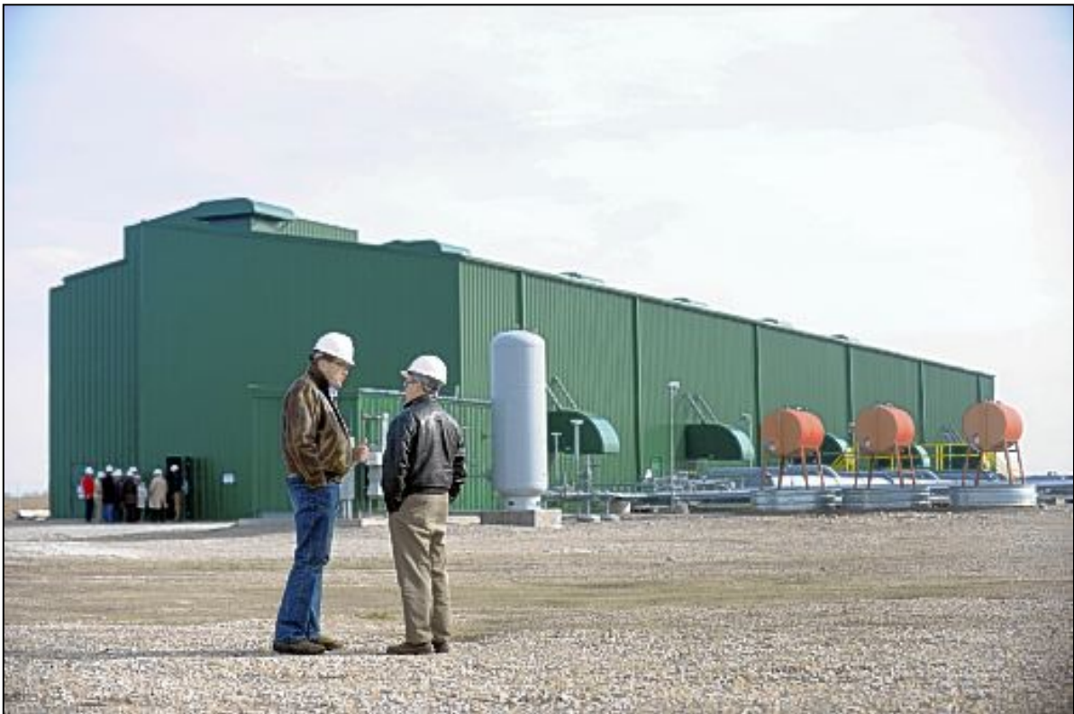
Gas Compressor Station
